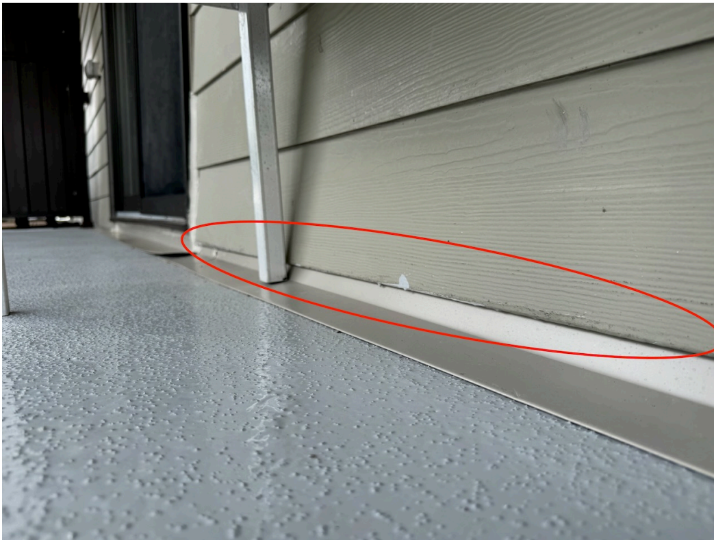
Photo 53: Clean and paint touch-ups required.
