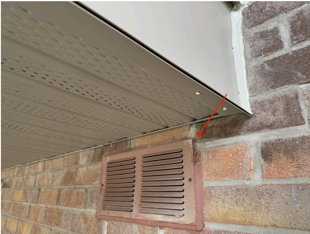
Photo 51: Caulking repairs required.
