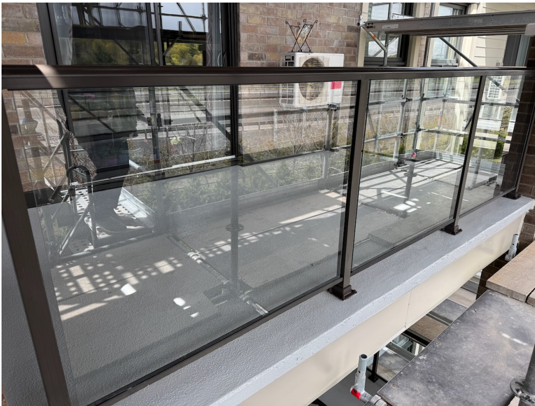
Photo 35: Masonry column cladding, flashing, caulking, and balcony traffic topping membrane complete. Guardrails re-installed.
