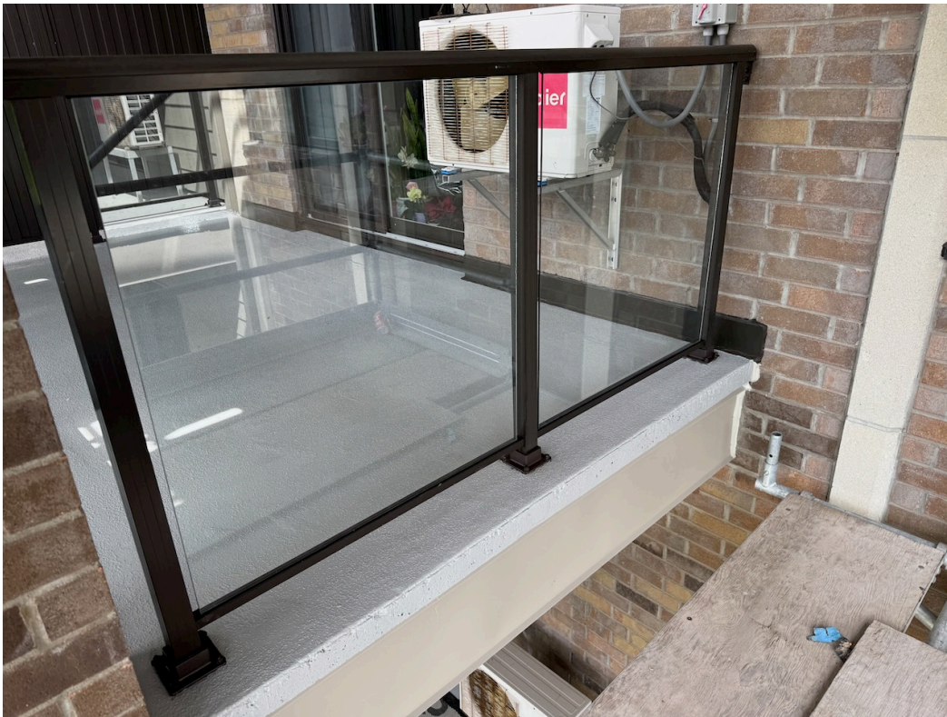
Photo 41: Masonry column cladding, flashing, caulking, and balcony traffic topping membrane complete. Guardrails re-installed.
