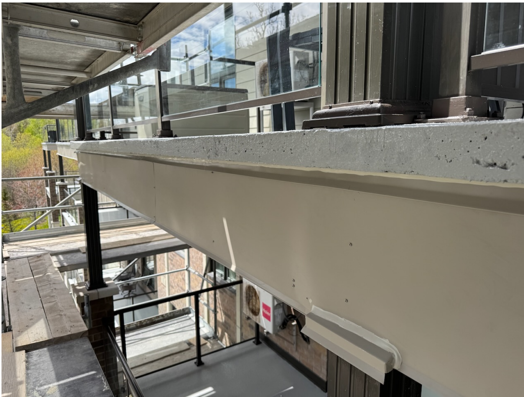
Photo 43: Aluminum column cladding, flashing, caulking, and balcony traffic topping membrane complete. Guardrails re-installed.
