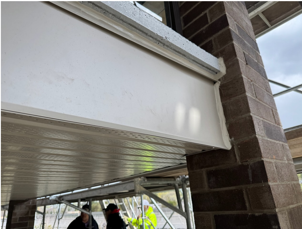
Photo 33: Masonry column cladding, flashing, caulking, and balcony traffic topping membrane complete. Guardrails re-installed.
