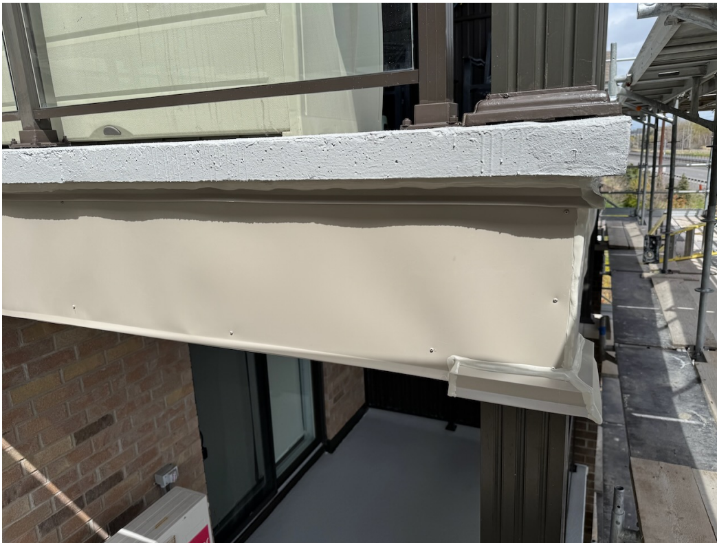
Photo 46: Aluminum column cladding, flashing, caulking, and balcony traffic topping membrane complete. Guardrails re-installed.
