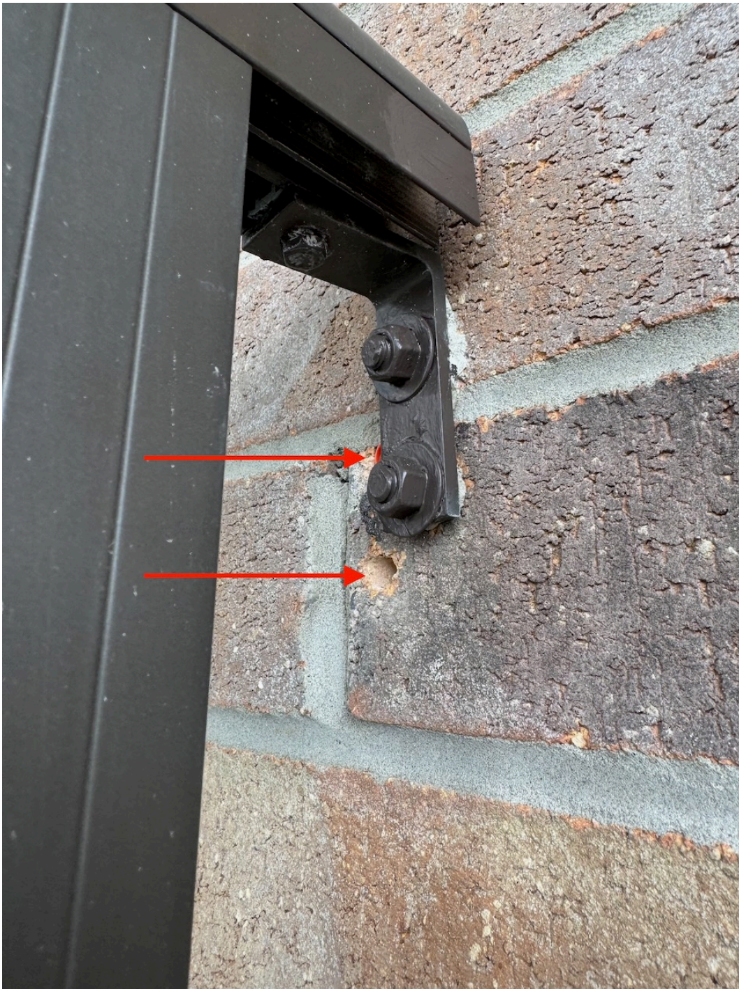
Photo 49: Caulking repairs required.
