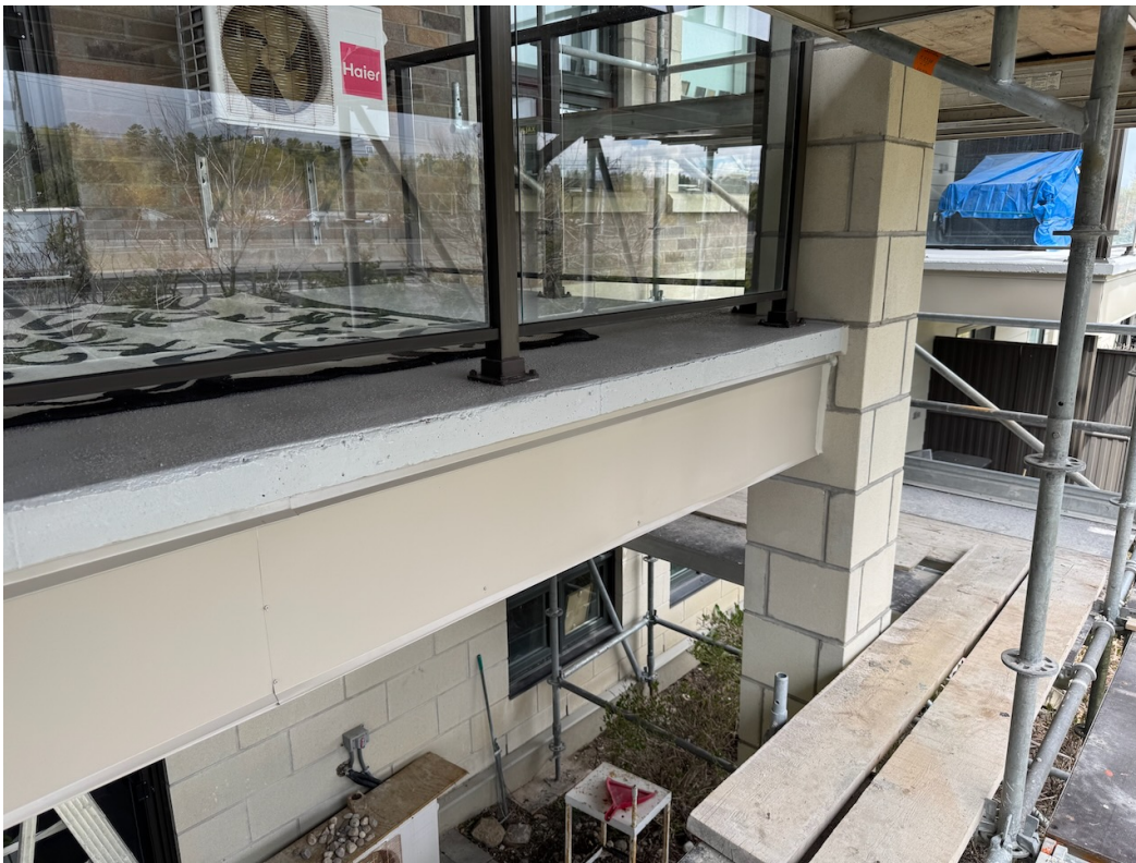
Photo 24: Masonry column cladding, flashing, caulking, and balcony traffic topping membrane complete. Guardrails re-installed.
