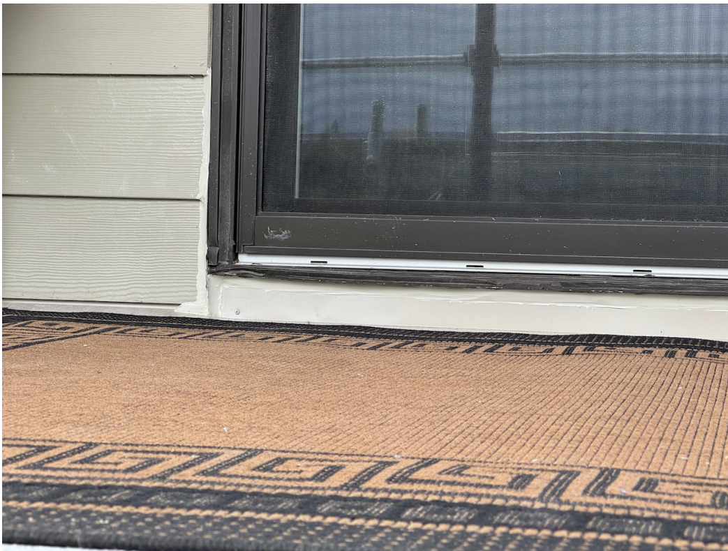
Photo 47: Caulking and flashing complete at the base wall around the patio door.
