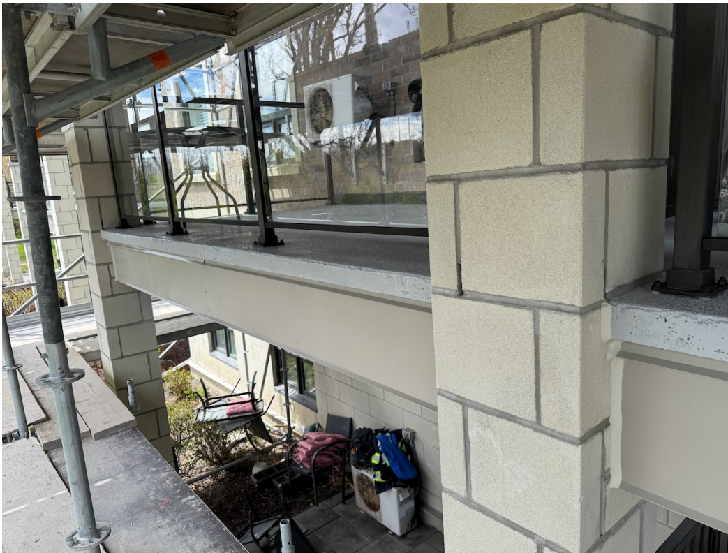
Photo 23: Masonry column cladding, flashing, caulking, and balcony traffic topping membrane complete. Guardrails re-installed.
