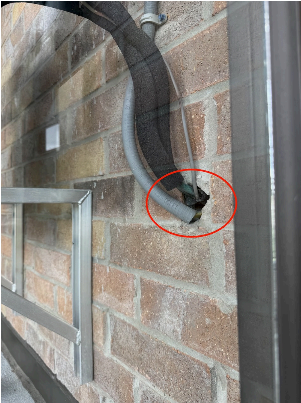
Photo 48: Caulking repairs required.
