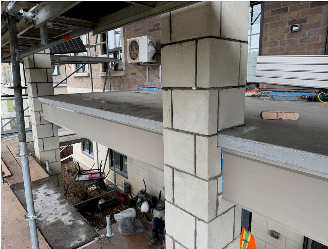
Photo 1: Drop 14 - April 30 - General view of the second floor balcony traffic topping, metal flashing, and masonry column cladding ongoing.
