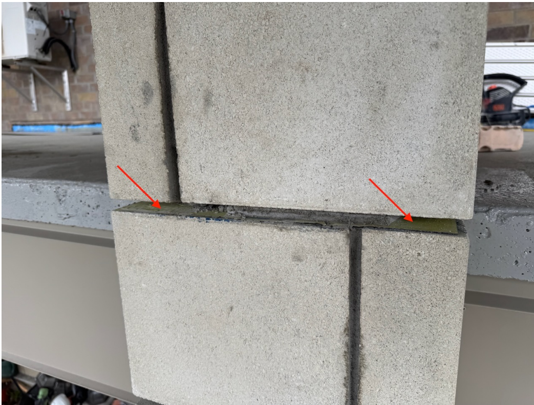
Photo 2: Blueskin TWF membrane installed at the balcony slab level through the masonry column cladding.
