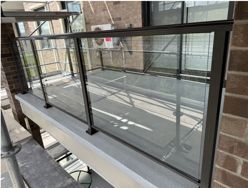
Photo 34: Masonry column cladding, flashing, caulking, and balcony traffic topping membrane complete. Guardrails re-installed.
