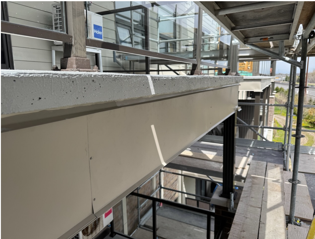
Photo 42: Aluminum column cladding, flashing, caulking, and balcony traffic topping membrane complete. Guardrails re-installed.
