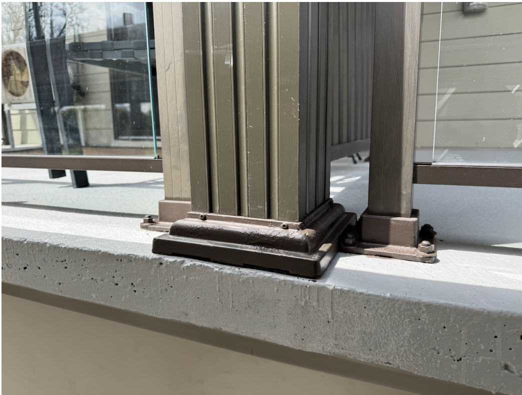
Photo 44: Aluminum column cladding, flashing, caulking, and balcony traffic topping membrane complete. Guardrails re-installed.
