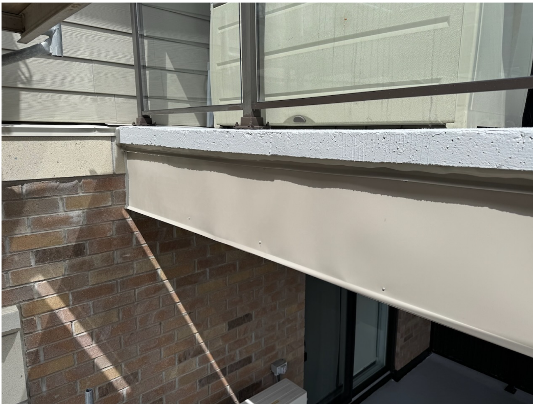
Photo 45: Aluminum column cladding, flashing, caulking, and balcony traffic topping membrane complete. Guardrails re-installed.
